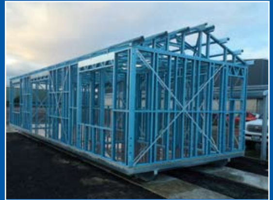
Framing system supplied, made from Bluescope steel.
